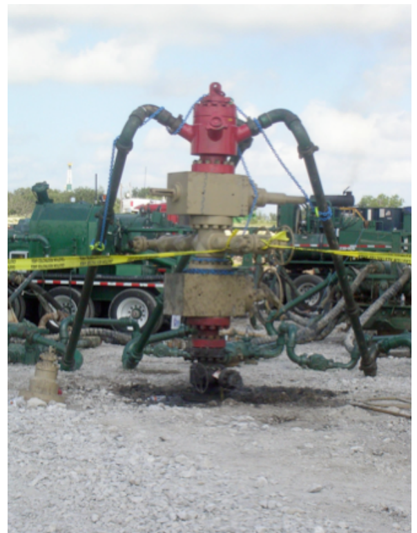
Figure 1 Not an alien probe—a wellhead for hydraulic fracturing, with injection pipes. (image: dpcusa.org)
